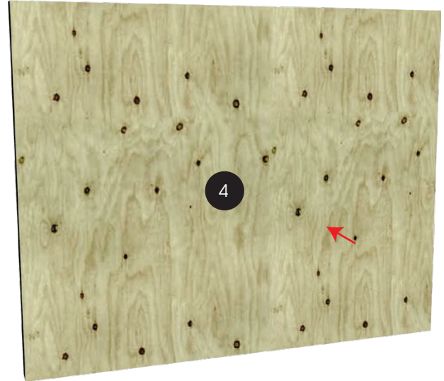
Install a layer of 15mm plywood (minimum CD grade) over top hats.
